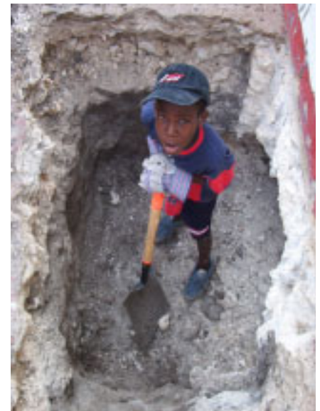
Boy from Bridgetown's Reed Street assists Canadian volunteer team in work on the foundation in January 2003.
